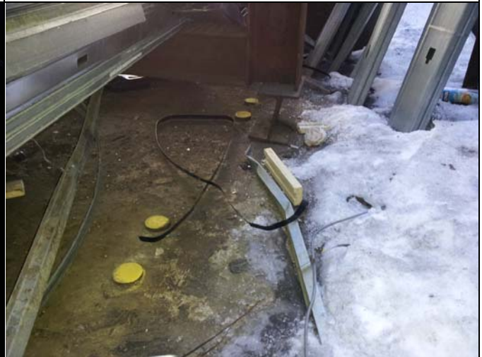
Two pairs of cut-off product/return lines to USTs
