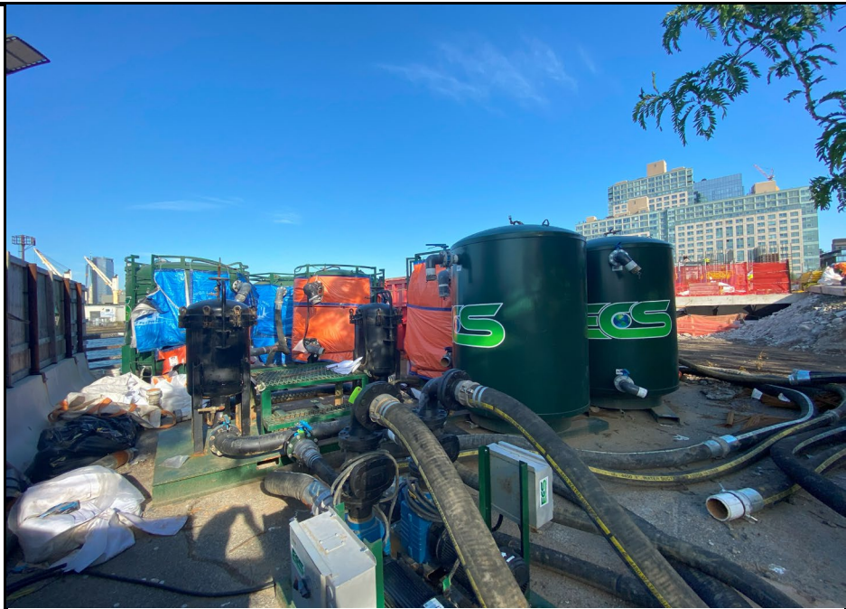
Photo 1: View of the maintainence on dewatering system.
