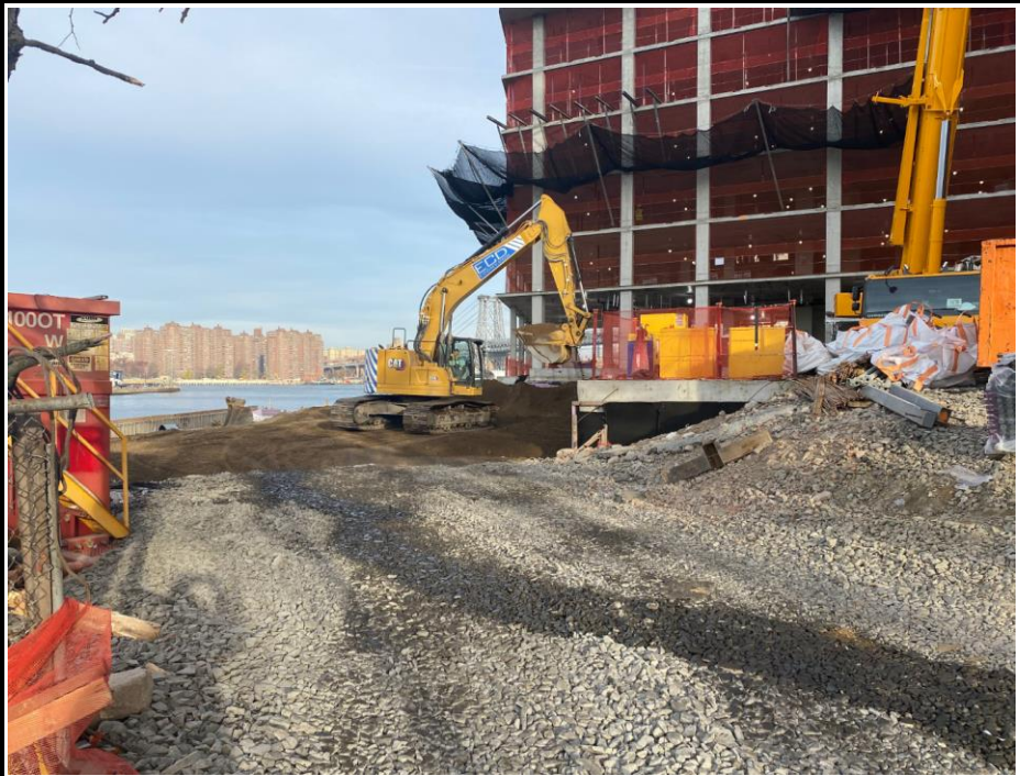
Photo 3: View of imported soil for use as general backfill in the marine area.
