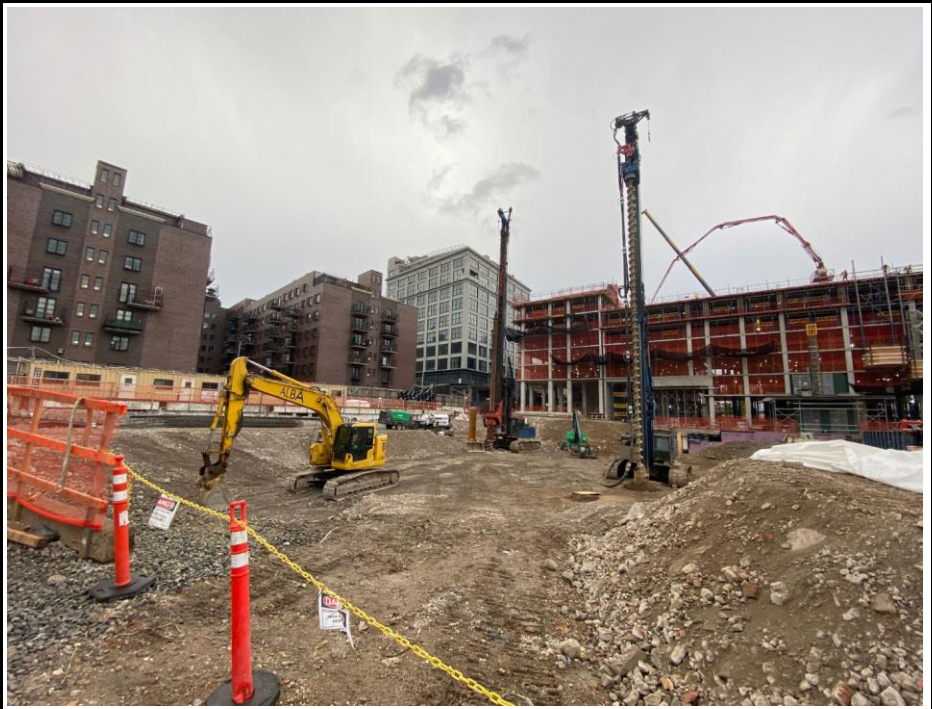
Photo 1: View of the Site and staged equipment facing southeast.
