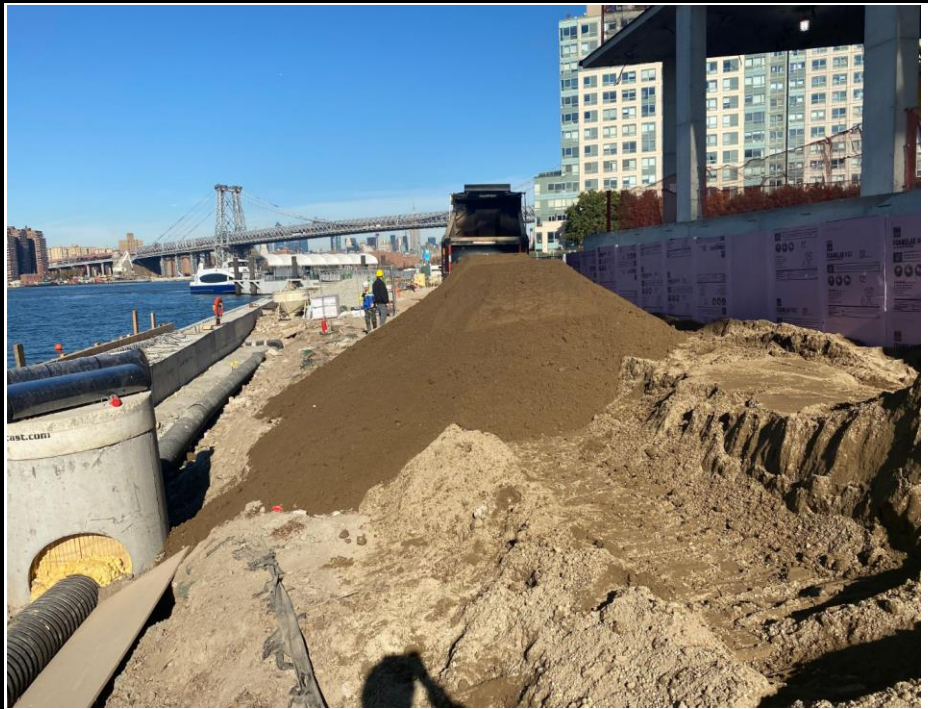
Photo 3: View of imported soil for use as general backfill in the marine area. .
