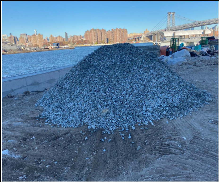
Photo 4: View of imported stone for use as bedding stone beneath the civil structures.
