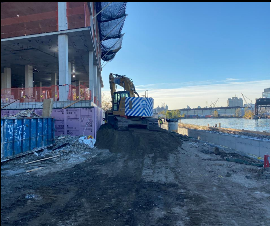
Photo 4: View of imported soil for use as general backfill in the marine area.
