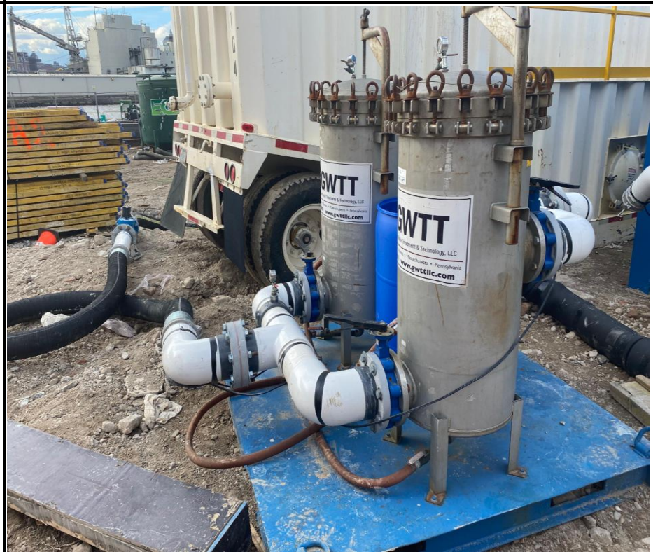
Photo 4: View of dewatering system equipment.
