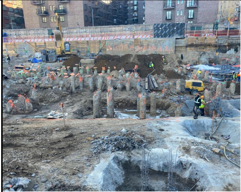
Photo 3: View of Site conditions and exposed piles facing east.
