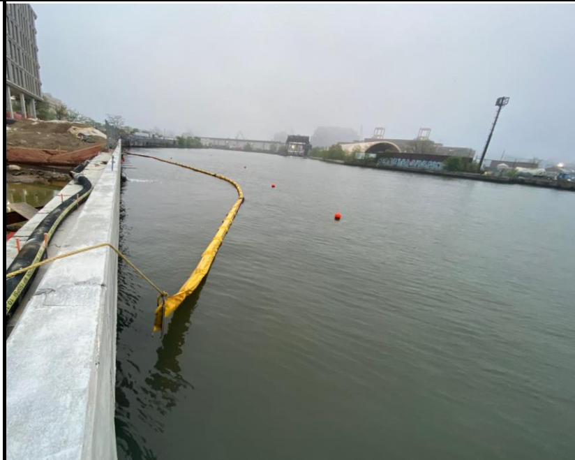
Photo 3: View of the dewatering effluent, following system maintenance completion.
