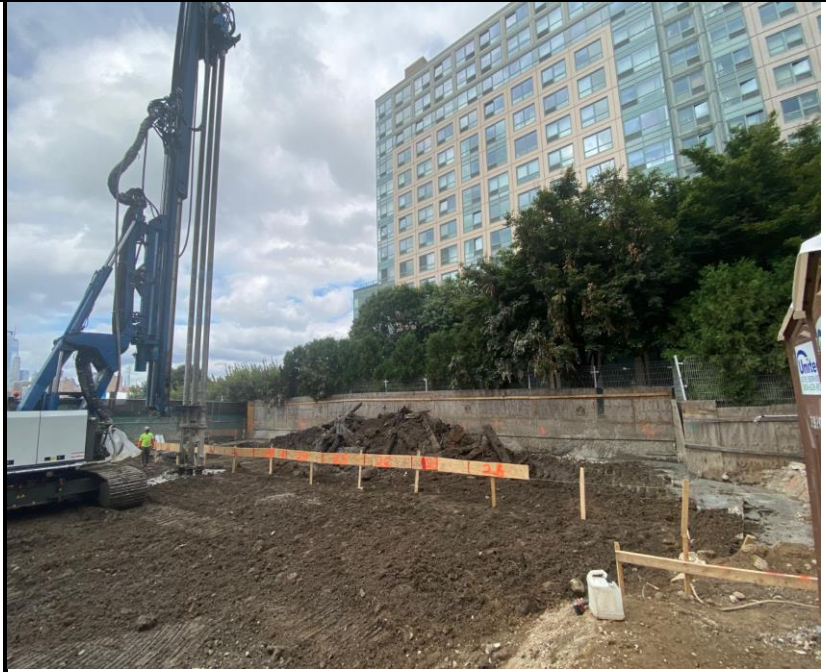
Photo 1: View of Site conditions, pile installation and map out of remedial excavation.
