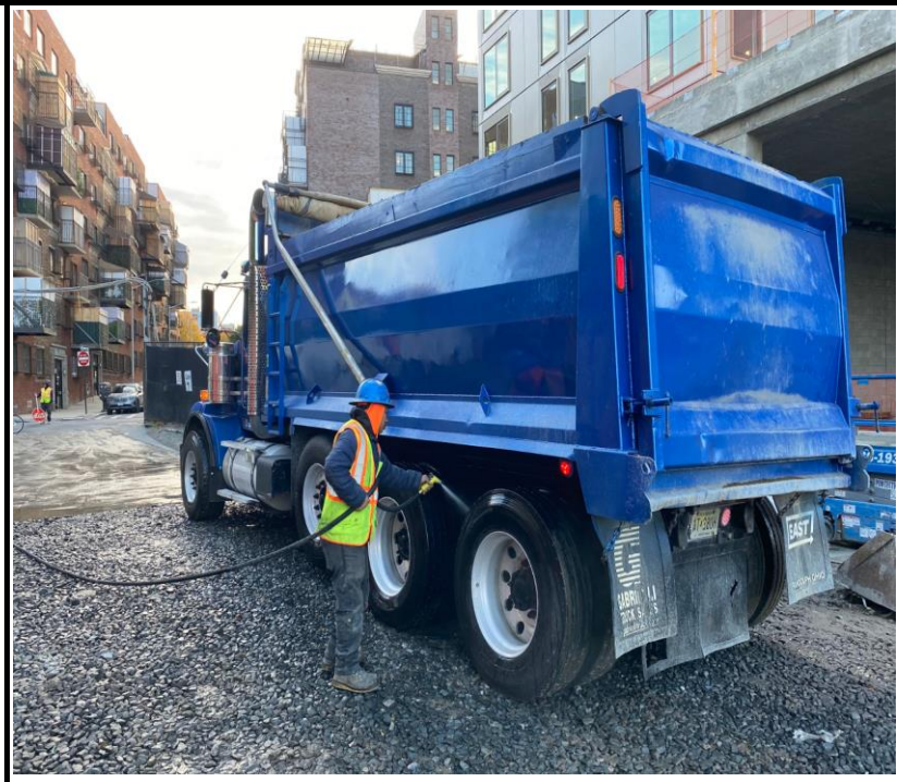
Photo 4: View of truck wash prior to trucks leaving the Site for off-site soil disposal.
