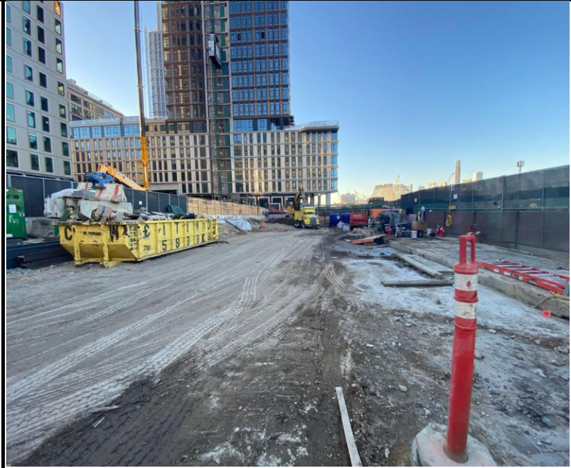
Photo 1: View of Site conditions and truck loading for off- site soil disposal facing south.
