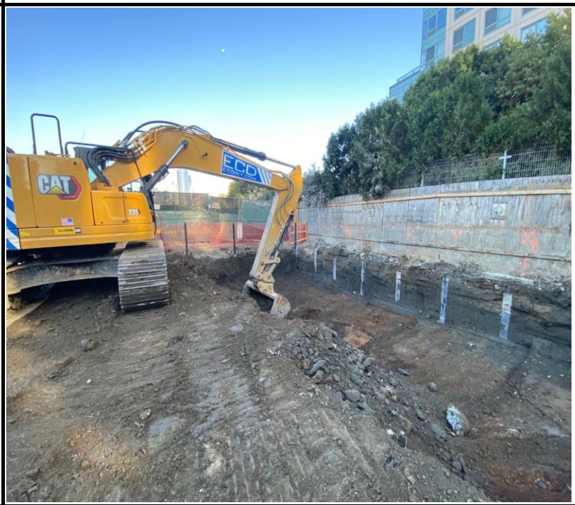
Photo 2: View of soil excavation in the northern remedial excavation, waste class grid WC-4.
