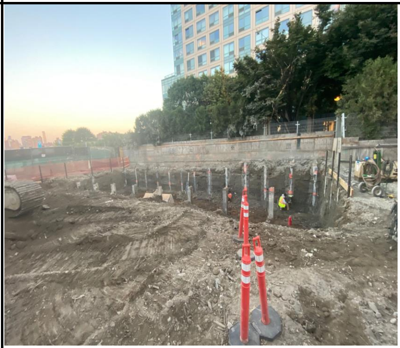
Photo 2: View of soil excavation in the northern remedial excavation, waste class grid WC-4.
