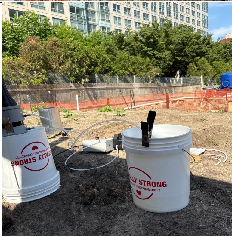
Photo 2: View of groundwater sampling.
