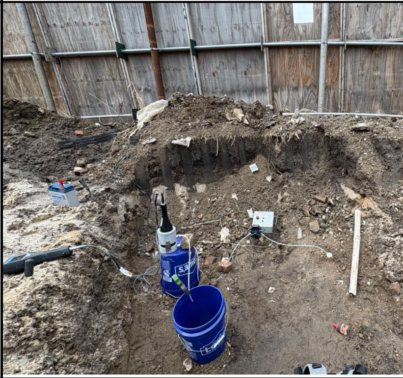
Photo 4: View of groundwater sampling.
