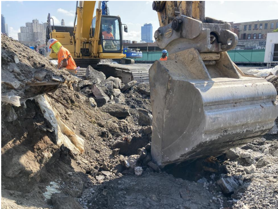
Photo 1: Kingdom excavating in the northern part of Society Brooklyn to facilitate collection of delineation samples (facing northeast)
