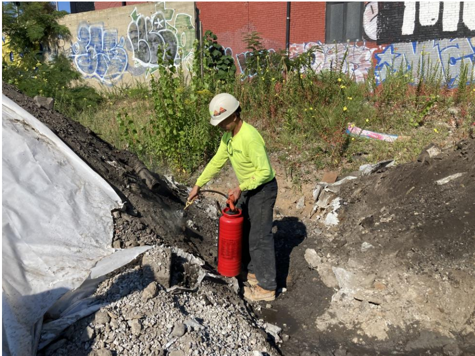
Photo 2: Kingdom applying odor suppressant (Biosolve Pinkwater) to the excavated soil in the southern part of Sackett Place (facing south)
