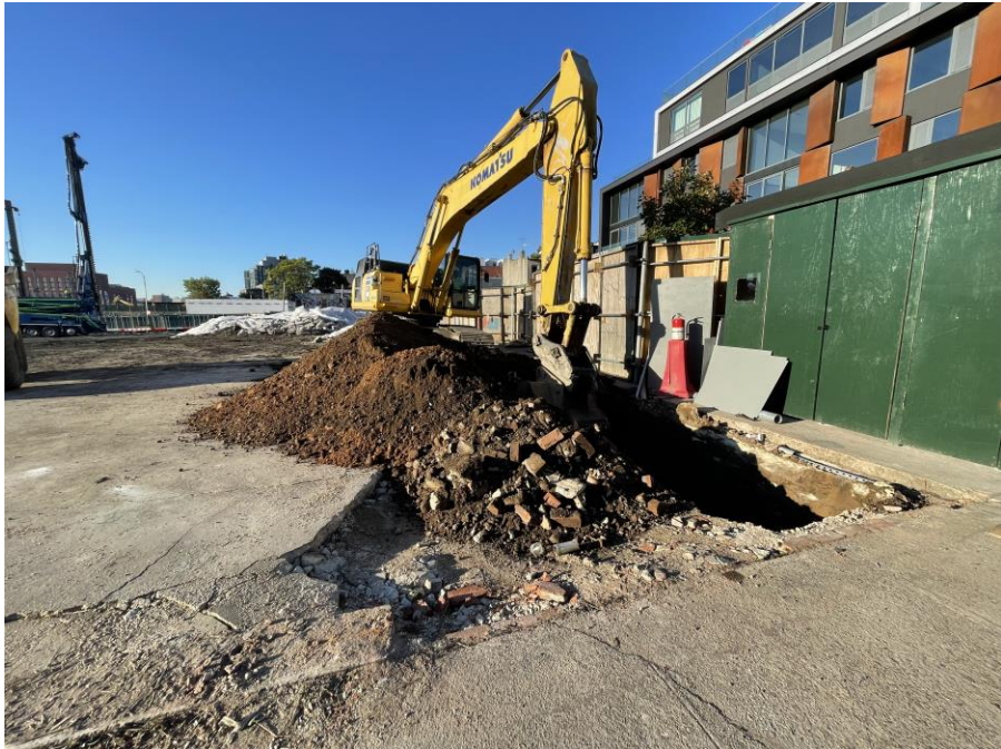
Photo 1: Kingdom excavating in the northwestern part of Society Brooklyn to pre-clear obstructions (facing southwest)
