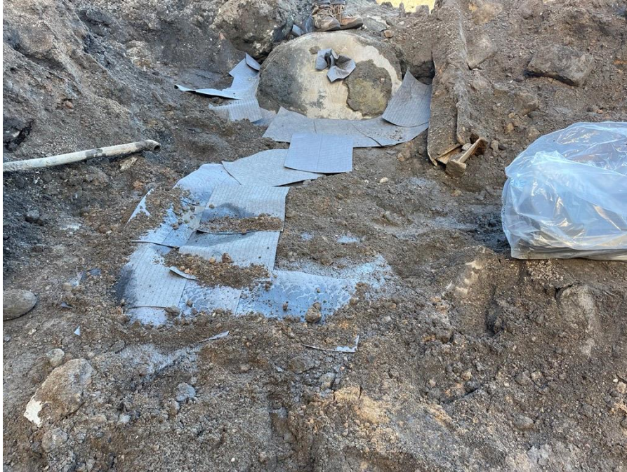
Photo 1: View of exposed 750-gallon UST and absorbent pads in the southwestern part of Sackett Place (facing north)
