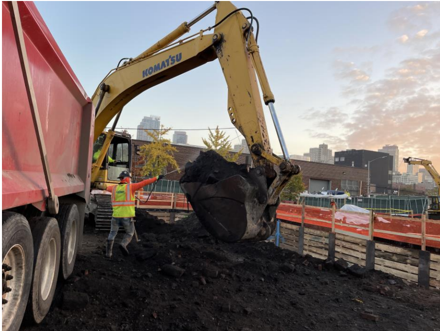
Photo 1: Kingdom applying Biosolve Pinkwater during excavation in the northern part of Society Brooklyn (facing east)
