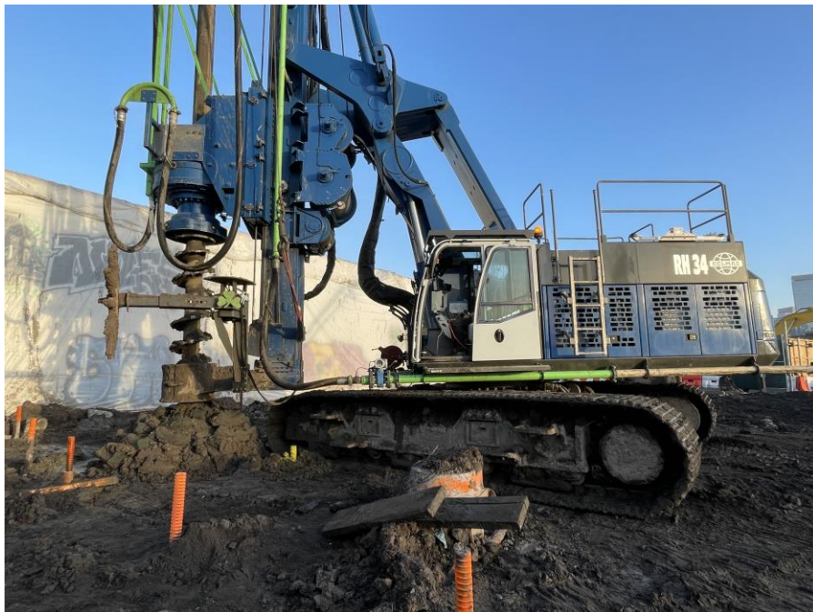
Photo 2: Kingdom installing a foundation pile in the western part of Sackett Place (facing north)
