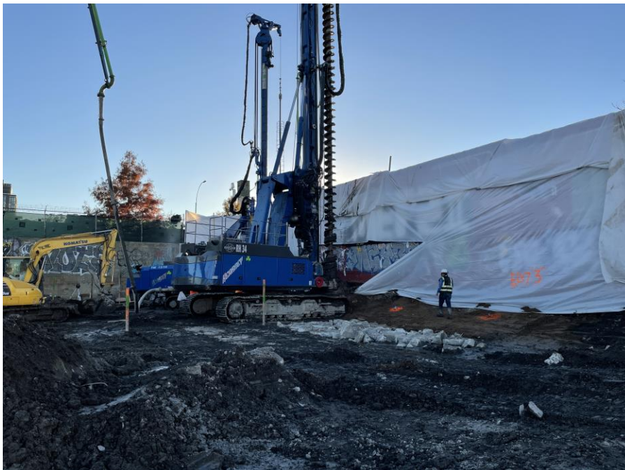
Photo 2: Kingdom installing foundation piles in the southwestern part of Sackett Place (facing southwest)
