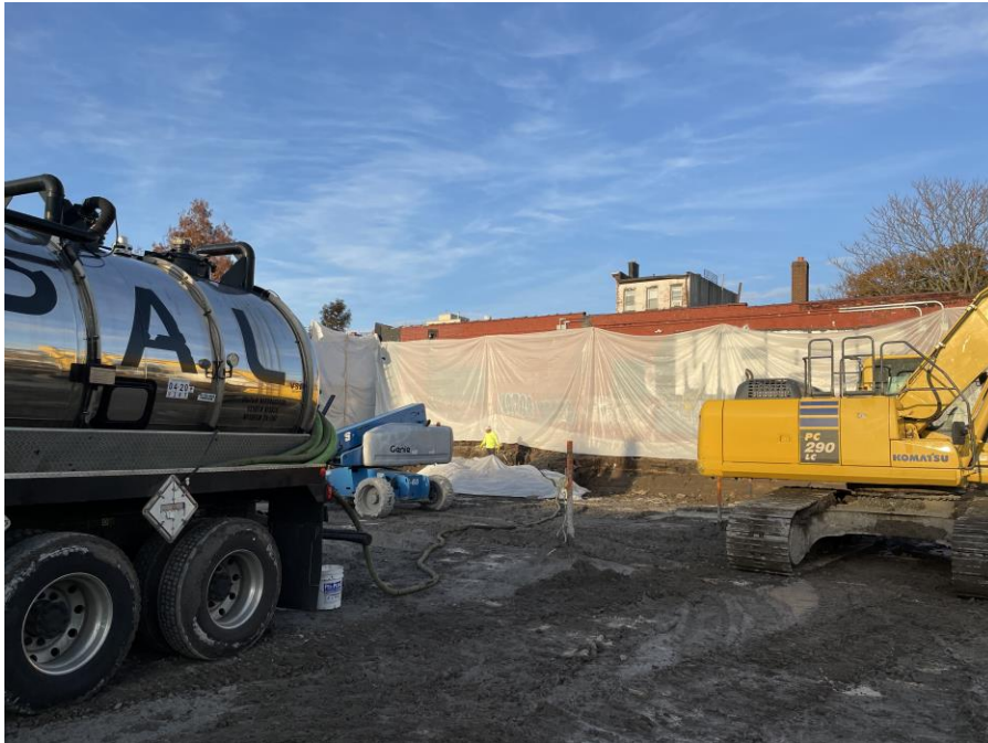
Photo 1: PAL vacuuming oily water into a permitted truck from the UST in the southwestern part of Sackett Place (facing southwest)
