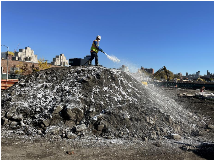
Photo 2: Kingdom applying ATMOS odor suppressant foam to a stockpile of petroleum-impacted soil/fill in the northern part of Society Brooklyn (facing northeast)
