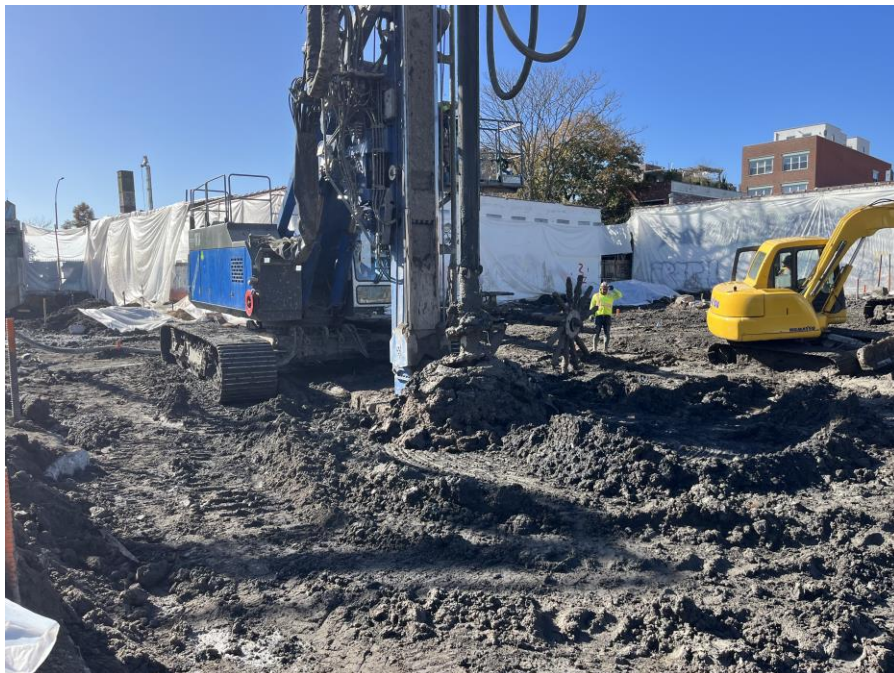
Photo 2: Kingdom installing foundation piles in the northern part of Sackett Place (facing southwest)
