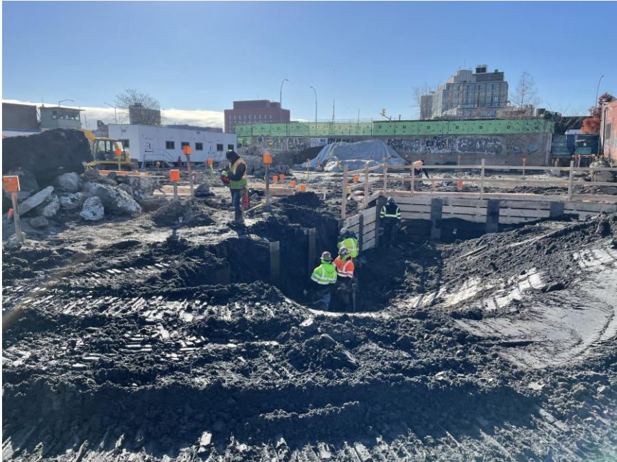
Photo 1: Kingdom installing lagging in the southern part of Sackett Street (facing southeast)
