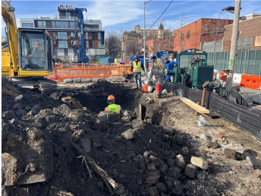
Photo 1: Kingdom applying Biosolve odor suppressant in the northern of Society Brooklyn (facing west)
