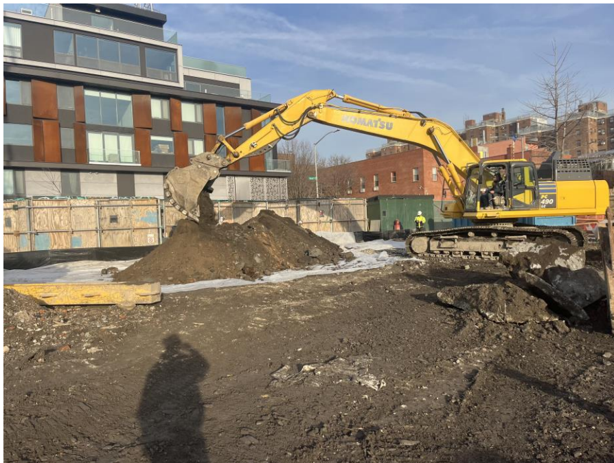
Photo 2: Kingdom excavating for pile cap load testing in the northwestern part of Society Brooklyn, and stockpiling historic fill on polyethylene sheeting (facing north)
