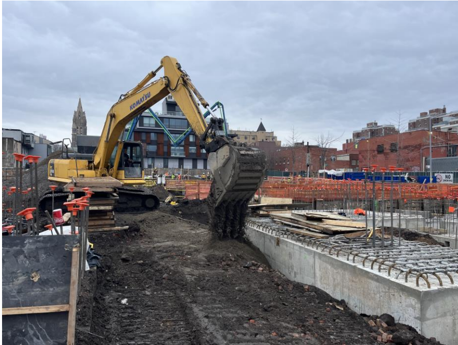
Photo 1: Kingdom backfilling around structural pile caps in the northeastern part of Society Brooklyn (facing northwest)
