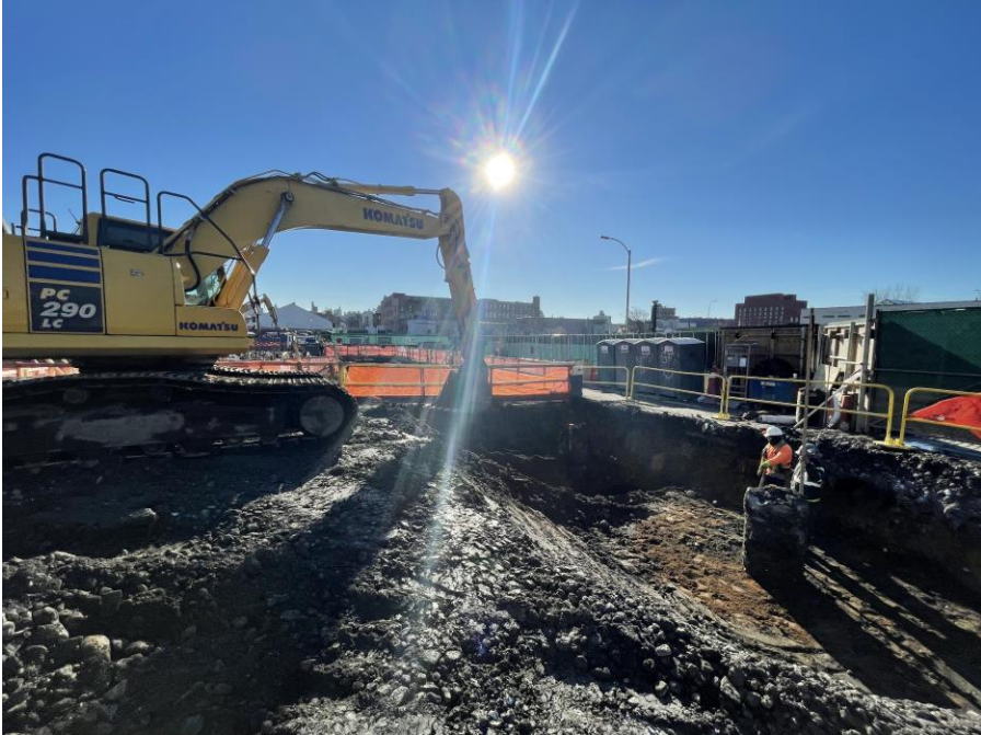
Photo 2: Kingdom excavating to install structural pile cap formwork in the southern part of Society Brooklyn (facing southeast)
