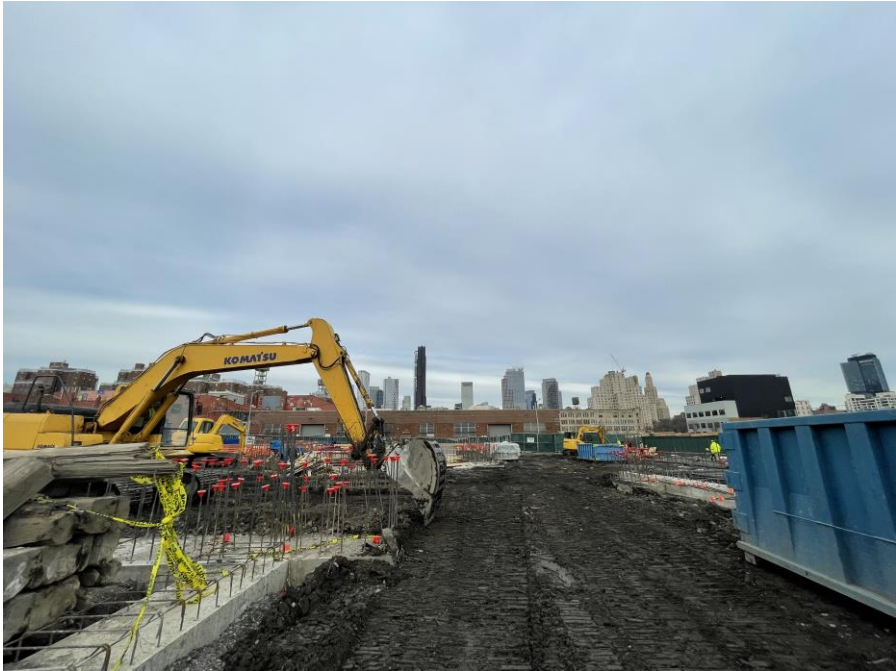
Photo 1: Kingdom backfilling to create a level working surface in the eastern part of Society Brooklyn (facing north)
