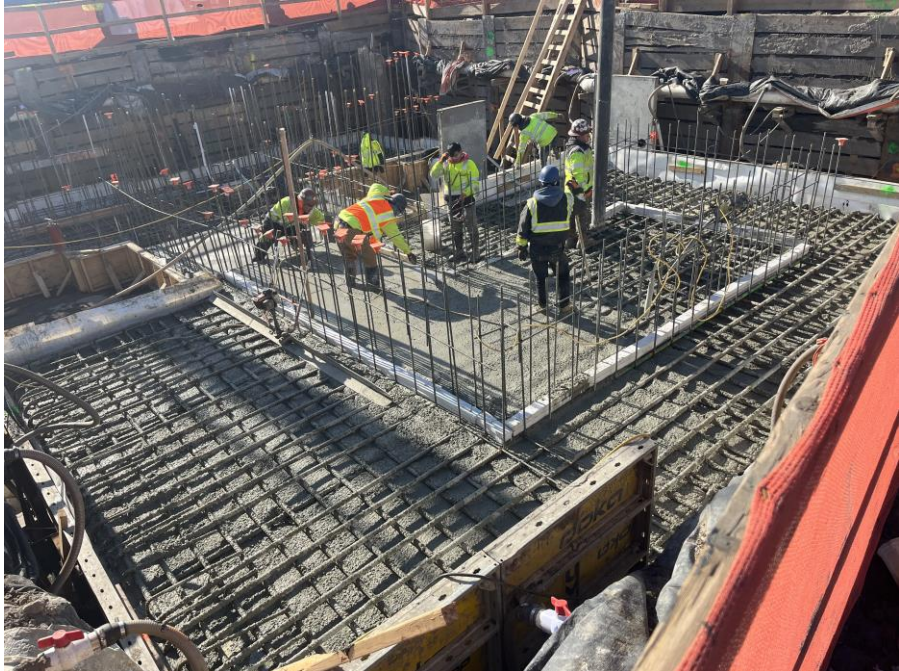
Photo 2: Kingdom placing concrete for the cellar-level foundation in the southern part of Society Brooklyn (facing southwest)
