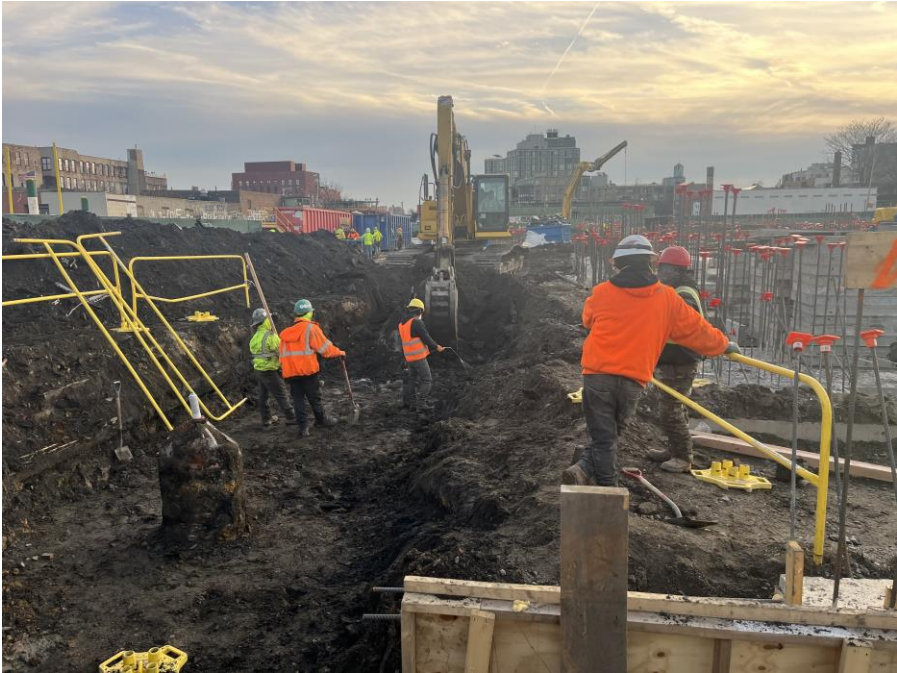
Photo 1: Kingdom excavating to install formwork in the northeastern part of Society Brooklyn (facing south)
