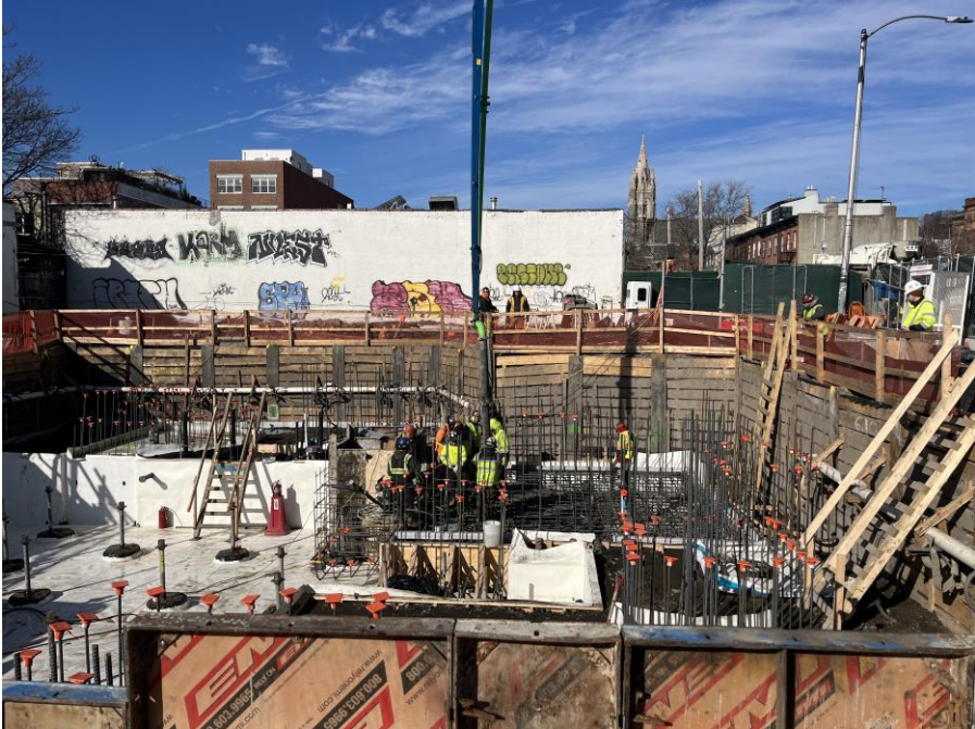
Photo 2: Kingdom placing concrete for the cellar-level foundation in the northern part of Sackett Place (facing west)
