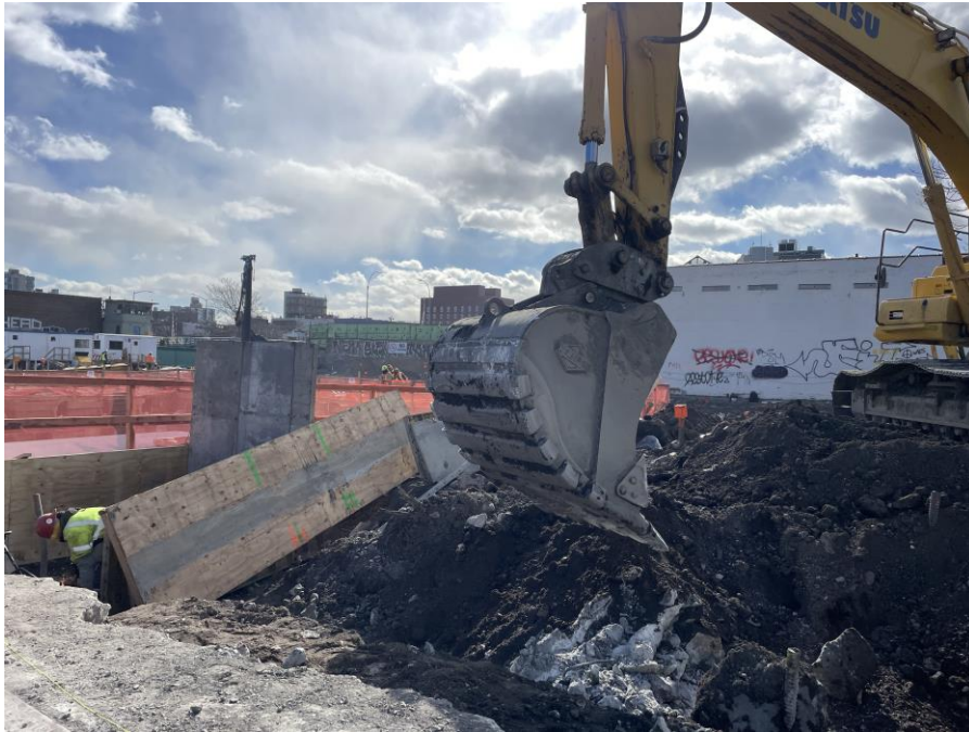
Photo 1: Kingdom excavating to install formwork in the northwestern part of Sackett Place (facing south)
