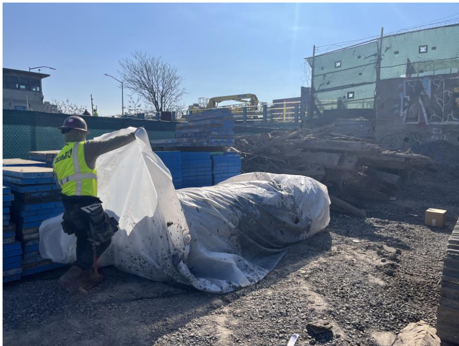
Photo 2: Kingdom covering a 550-gallon UST with polyethylene sheeting in the southeastern part of Sackett Place (facing southeast)
