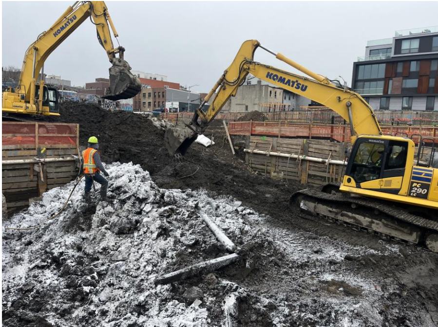
Photo 2: Kingdom applying ATMOS odor suppressant foam in the northern part of Society Brooklyn (facing southwest)
