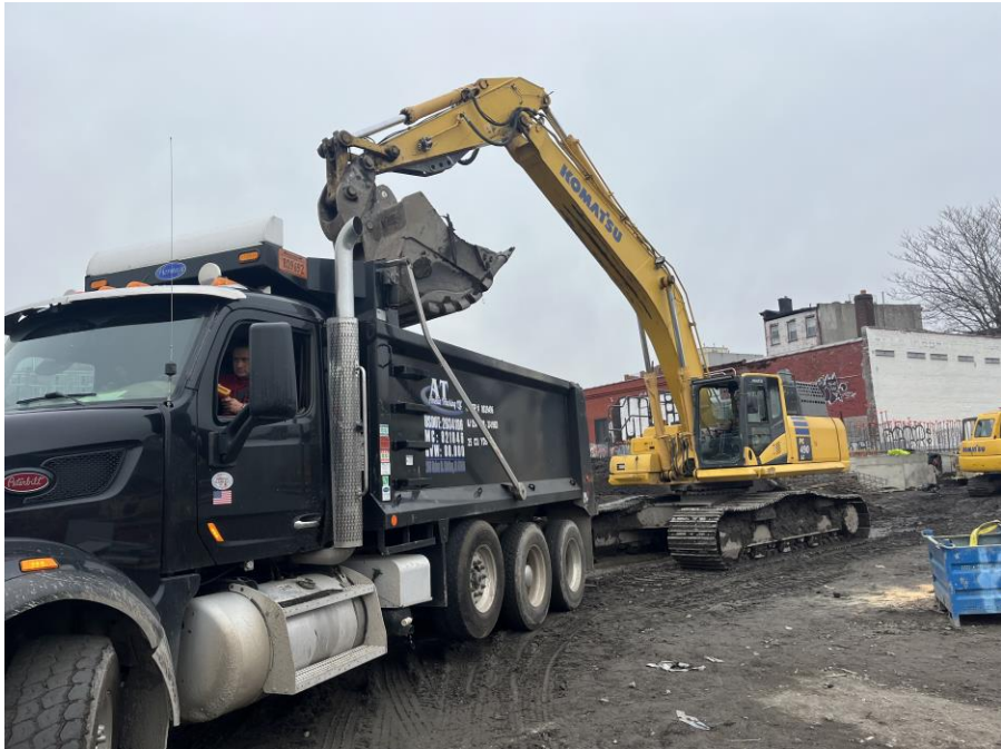
Photo 1: Kingdom exporting non-hazardous historic fill in permitted tri-axle trucks in the southern part of Sackett Place (facing southwest)
