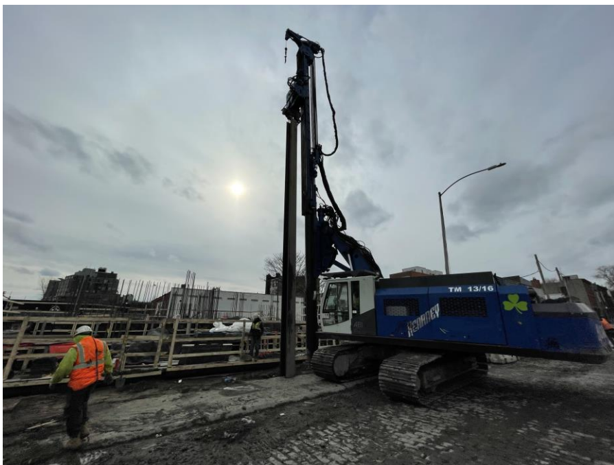
Photo 2: Kingdom removing soldier pile in the northern part of Sackett Place (facing southwest)
