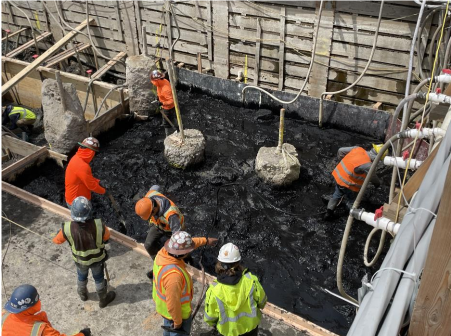
Photo 1: Kingdom applying Petrofix reagent to the base of Remedial Excavation Area No. 1 in the northern part of Society Brooklyn (facing west)
