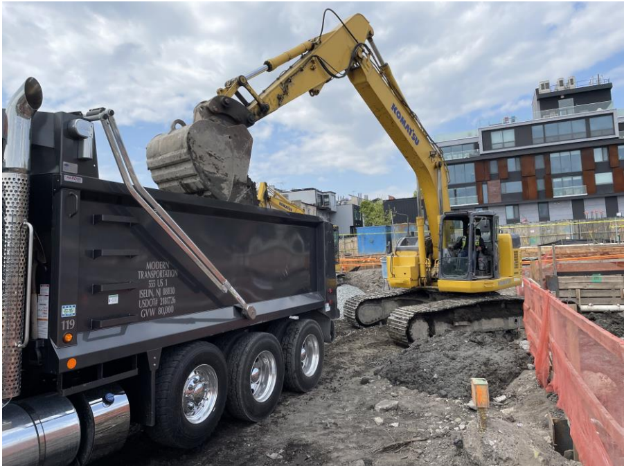
Photo 2: Kingdom exporting non-hazardous soil/fill in permitted tri-axle trucks in the northern part of Society Brooklyn (facing west)
