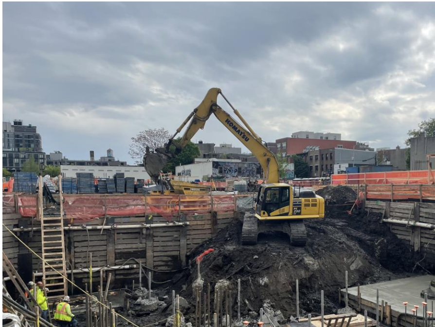
Photo 2: Kingdom excavating for the future cellar in the northern part of Society Brooklyn (facing southwest)
