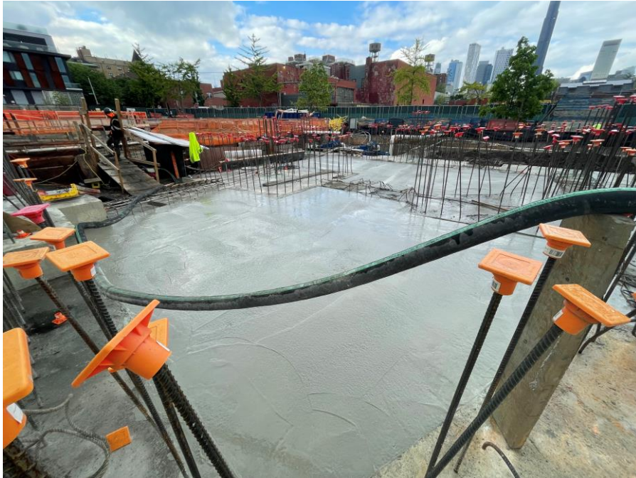
Photo 1: Kingdom placing concrete for a mud slab above the SMD system in the northeastern part of Society Brooklyn (facing northwest)
