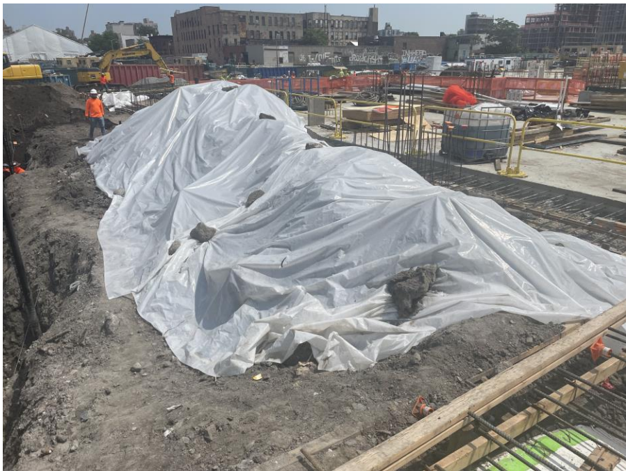
Photo 2: Stockpiled historic fill/soil in the central part of Society Brooklyn (facing southeast)
