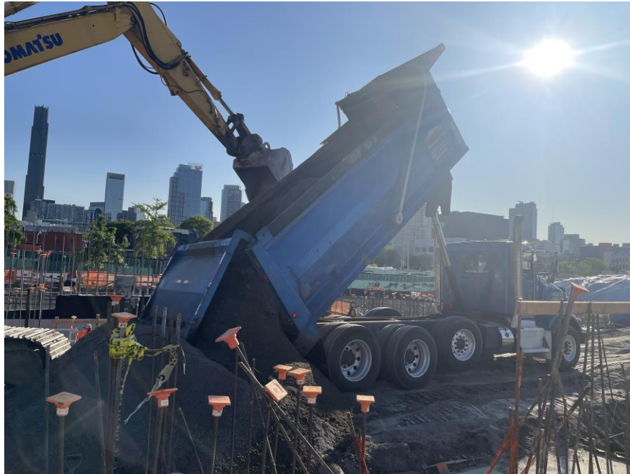
Photo 1: Kingdom importing 0.5-inch crushed stone in the central part of Society Brooklyn (facing northeast)
