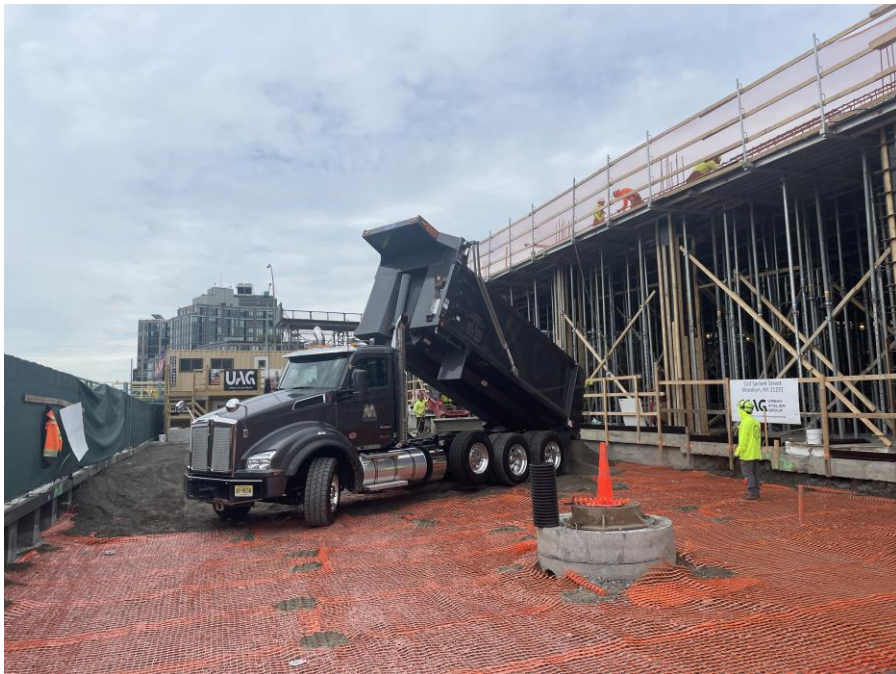
Photo 2: G&M importing 0.5-Inch crushed stone for the temporary composite cover system in the southeastern part of Sackett Place within the SPW (facing southwest)
