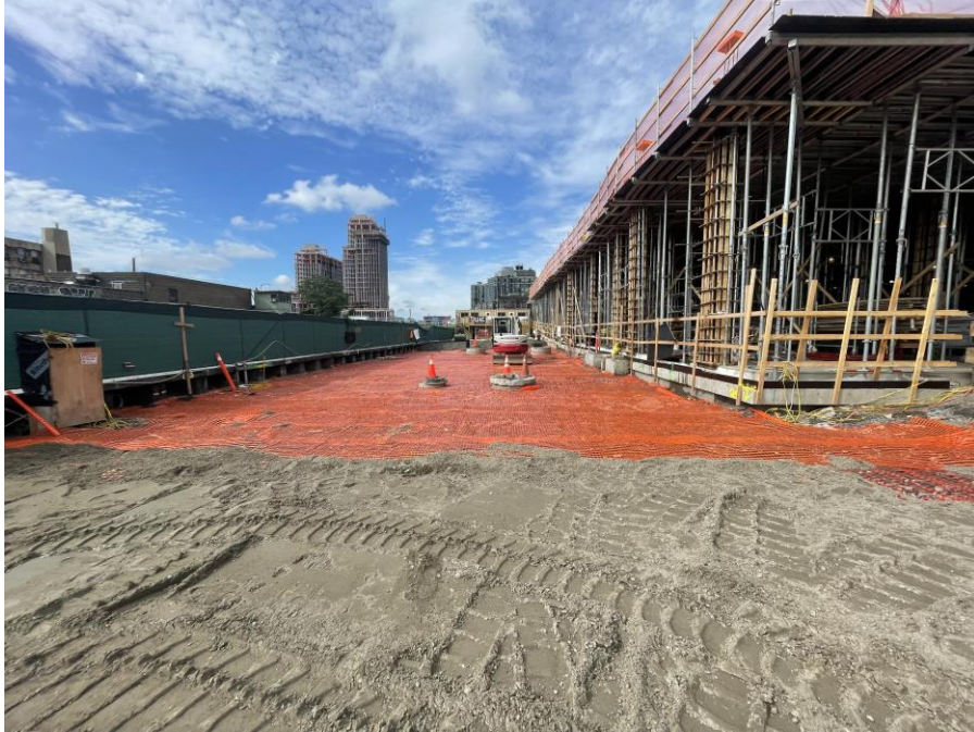
Photo 1: G&M installing demarcation layer as part of the temporary composite cover system in the southeastern part of Sackett Place within the SPW (facing south)
