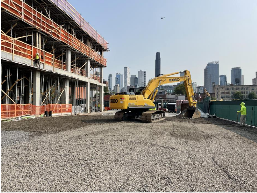
Photo 1: G&M placing 0.75-inch crushed stone for the temporary composite cover system in the northeastern part of Society Brooklyn (facing northeast)
