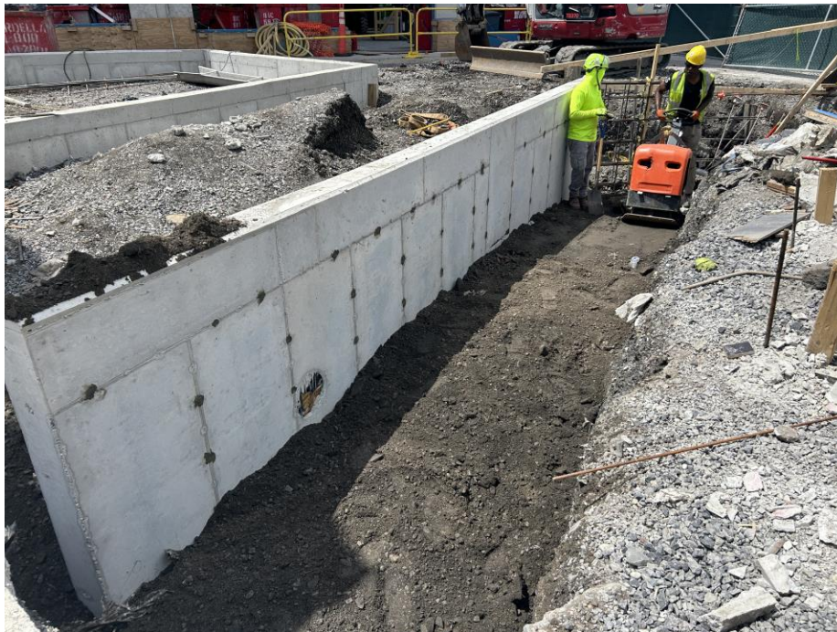
Photo 2: G&M backfilling in the northeastern part of Society Brooklyn within the SPW (facing north)
