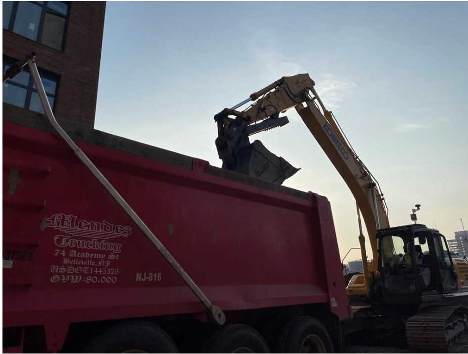
Photo 1: G&M exporting non-hazardous historic fill/soil in permitted tri-axle trucks from Society Brooklyn (facing northeast)
