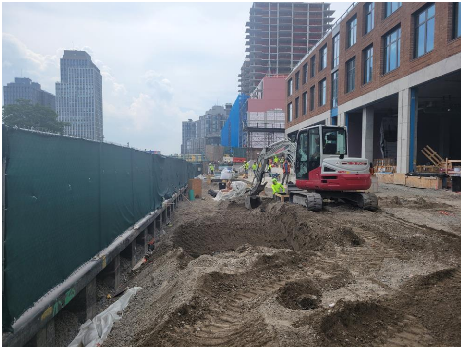
Photo 2: G&M excavating in the eastern part of the SPW in Sackett Place (facing south)
