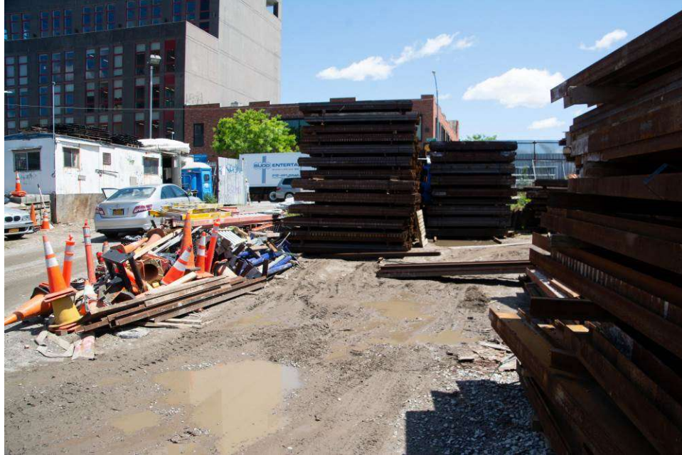
Condition of yard near SV-6; entrance ramp in background
