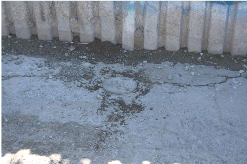
Photo from 2018 showing deterioration of sidewalk and MW-7 in Boerum Street
