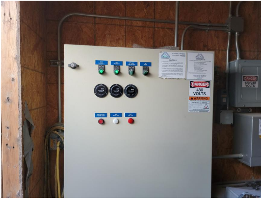
SVE System functioning
