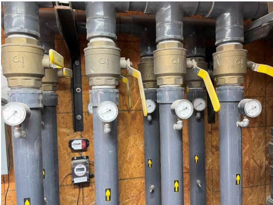
DESCRIPTION: SVE Piping
