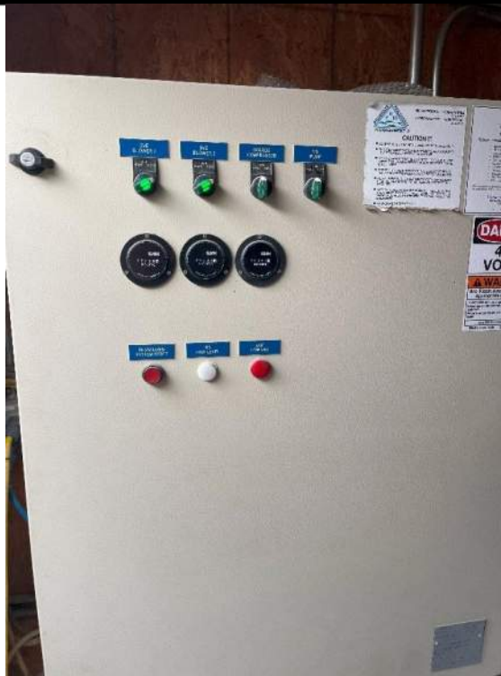
DESCRIPTION: SVE Control Panel
