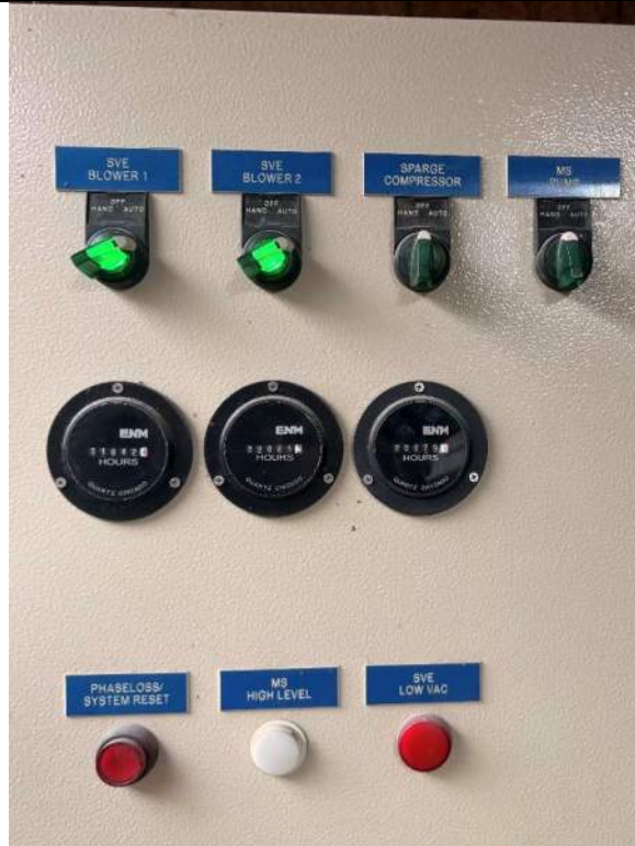
Description: SVE Control Panel
