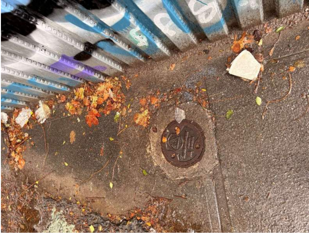
Description: MW-8 Located on McKibbin Street.
