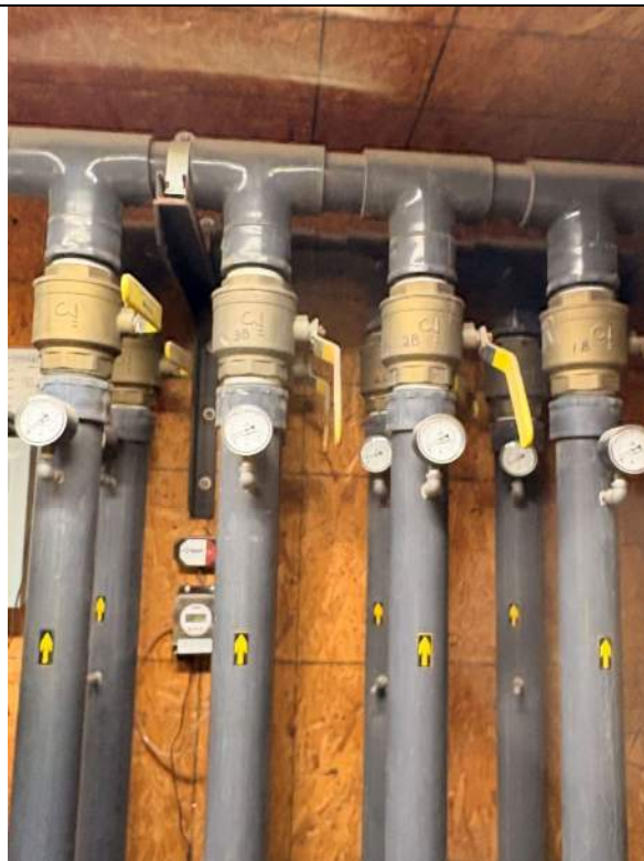
Description: SVE Piping
