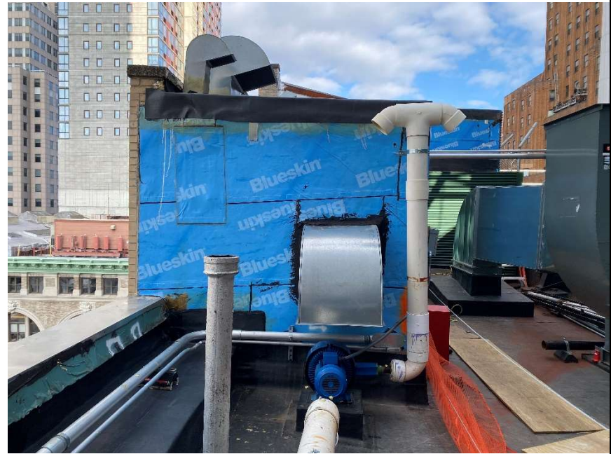
Photo 14: Modified blower and exhaust stack location.
