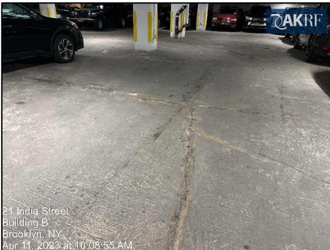
Photograph 11: Sealed surficial cracks observed in Building B floor slab.
