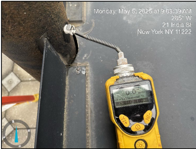
Photograph 1: Exhaust riser pipe sample port PID measurement.
