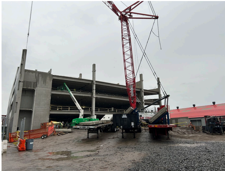
Photo 1: Facing south, delivery of preformed concrete to site and superstructure status at beginning of day.
