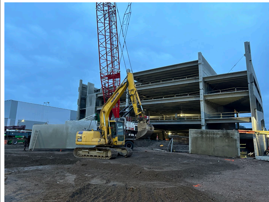
Photo 4: Superstructure status at the end of the day and crane pad leveling.
