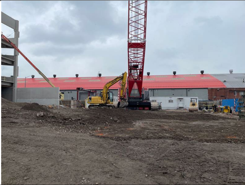
Photo 3: Looking west, progress of excavation and grading in grids A1 and B1.
