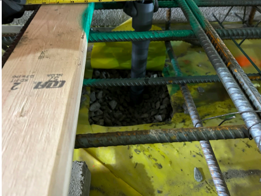
Photo 3: Southernmost SSDS monitoring point is being installed in the permeable subbase layer in grid A4.
