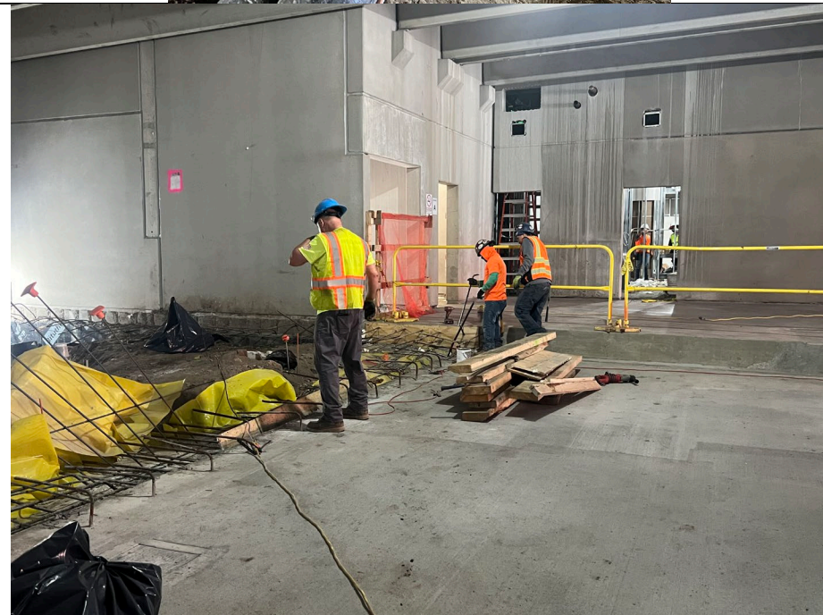
Photo 4: Looking east, view of rebar maintenance at the end of previously poured section of foundation slab.
