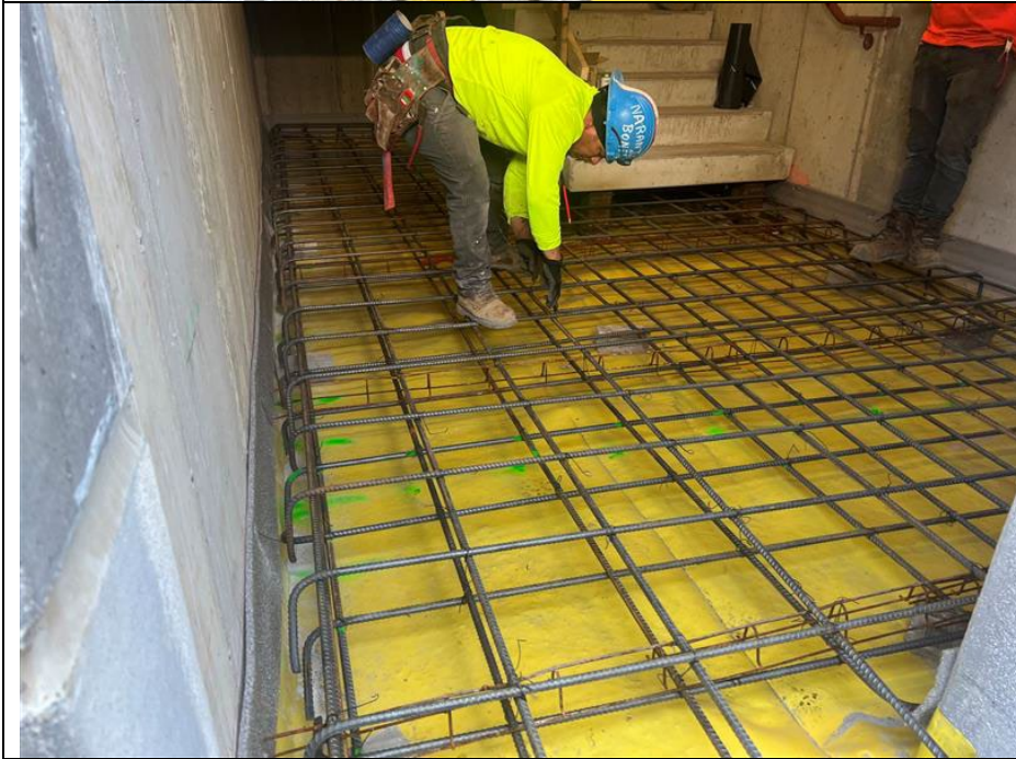
Photo 2: Looking west, Kingdom adding rebar in staircase landing B in preparation for pour.
