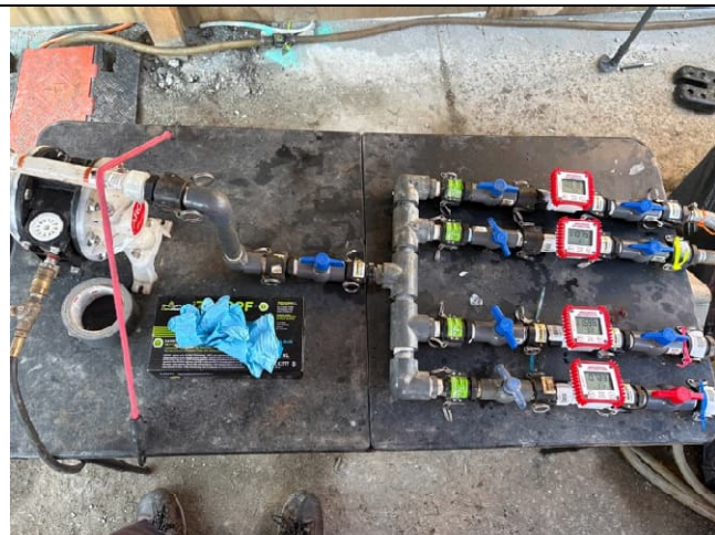
Photo 4 – Pump and flow/volume meters
