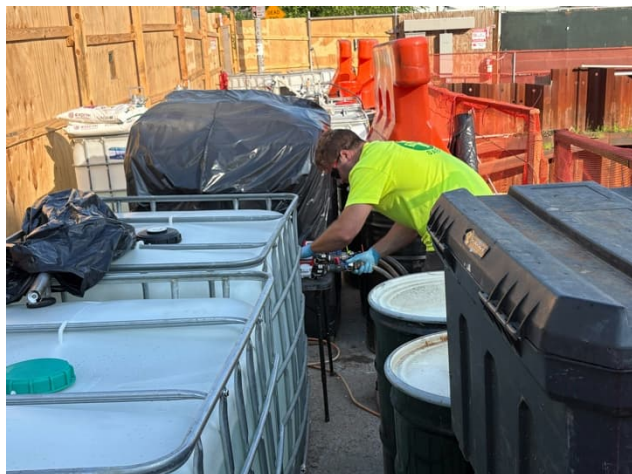
Photo 1 – Hookup of tubing to pump manifold.
