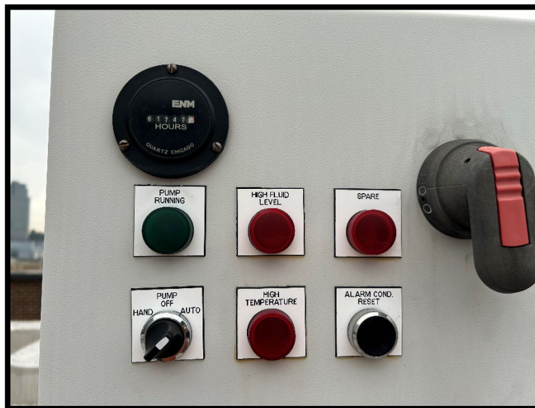
Photograph 10: View of SSDS Blower 1 (west) control panel; green pilot light bulb is out; other indicators show system is operational.
