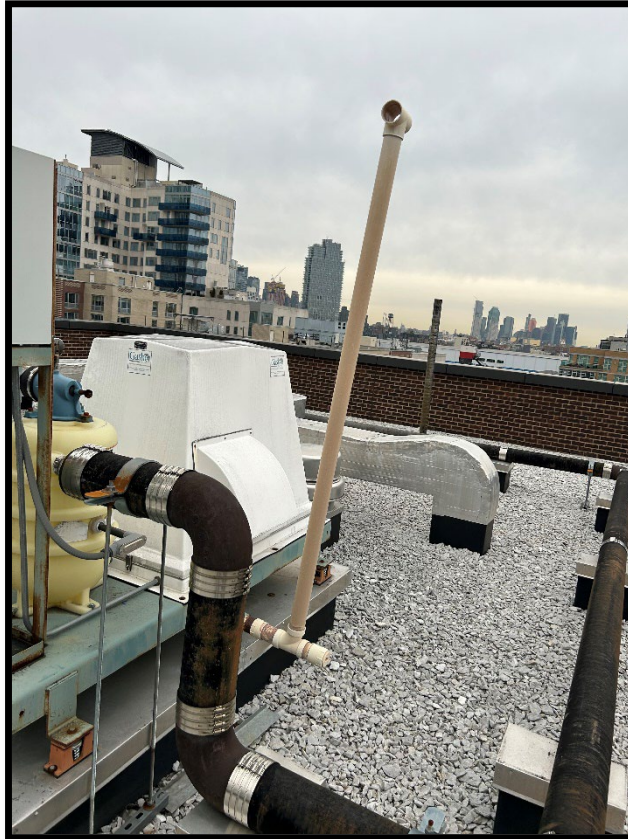
Photograph 11: SSDS Blower 1 (west) air inlet filters and knock out tank in view.
