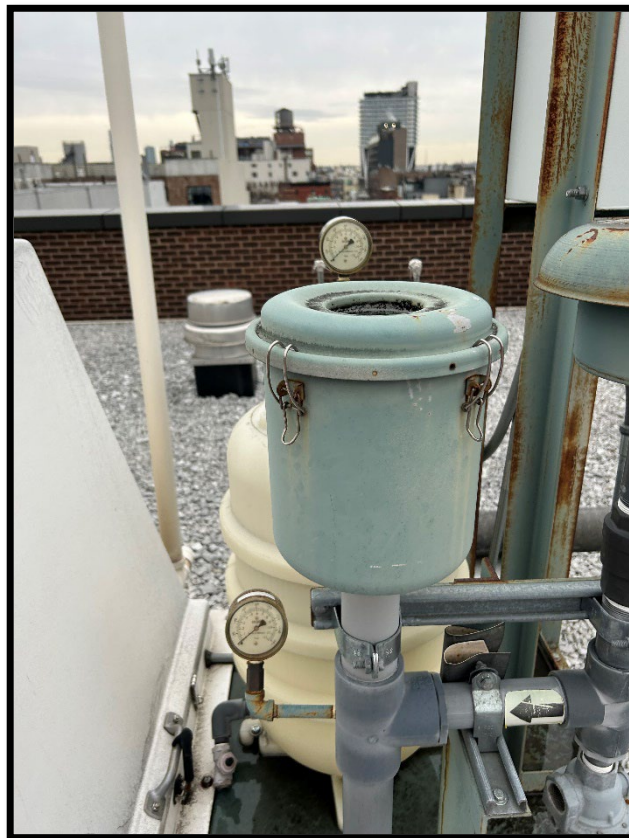
Photograph 16: Photo of SSDS Blower 2 (east) inlet filter and gauges.
