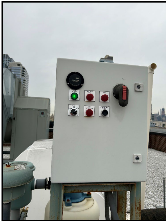
Photograph 14: Photo of SSDS Blower 2 (east) control panel.
