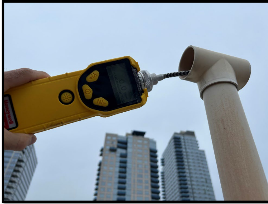
Photograph 9: View of 0.0ppm PID reading at SSDS Blower 1 (west).
