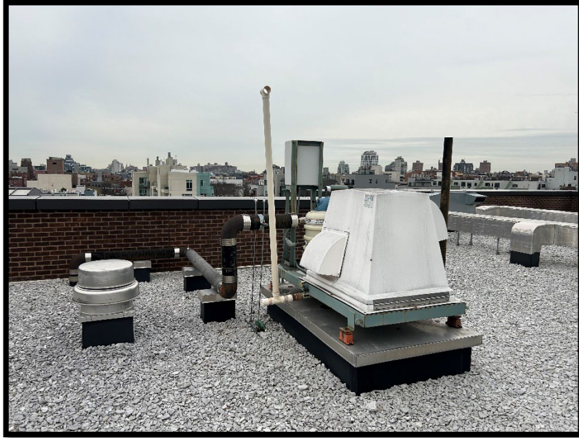
Photograph 15: Photo of the SSDS Blower 2 (east) configuration.
