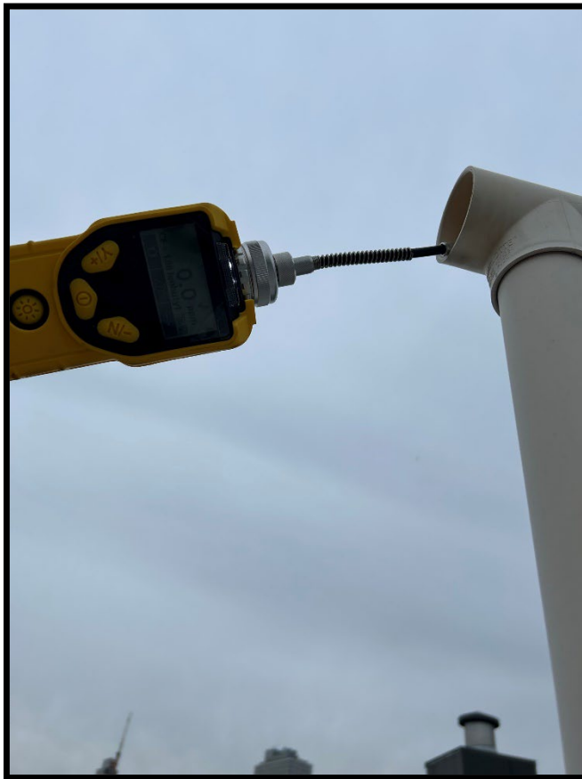
Photograph 13: View of 0.0ppm PID reading at SSDS Blower 2 (east).
