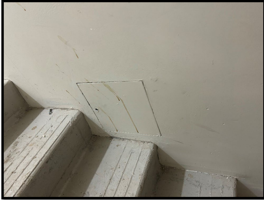
Photograph 7: Photo of lock box containing MP-1 (west SSDS) within stairwell between first floor to the cellar.
