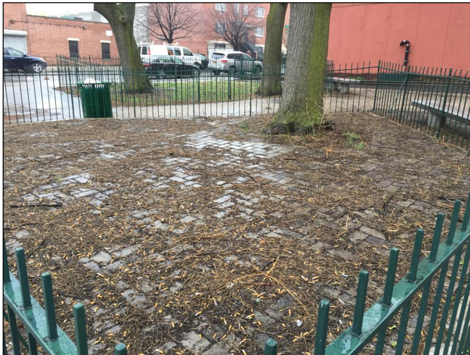
Photo 3: Looking northwest at porous paving installed at Site; twigs, leaves, and twigs present.
