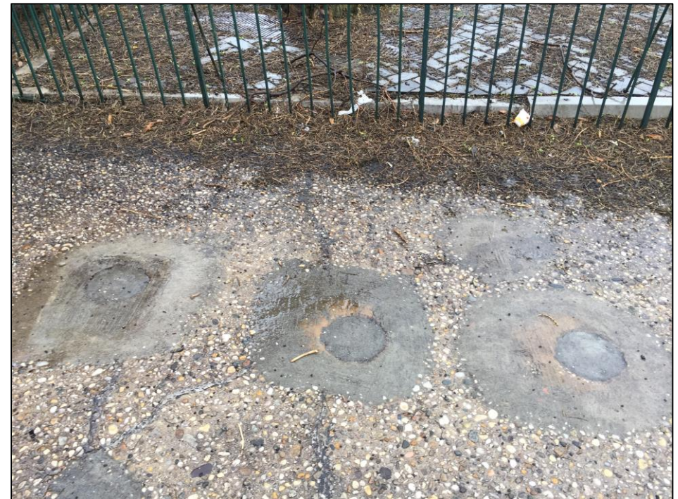
Photo 8: Repaired soil borings/soil vapor sampling locations. No cracks in surrounding concrete sidewalk; no repairs necessary.
