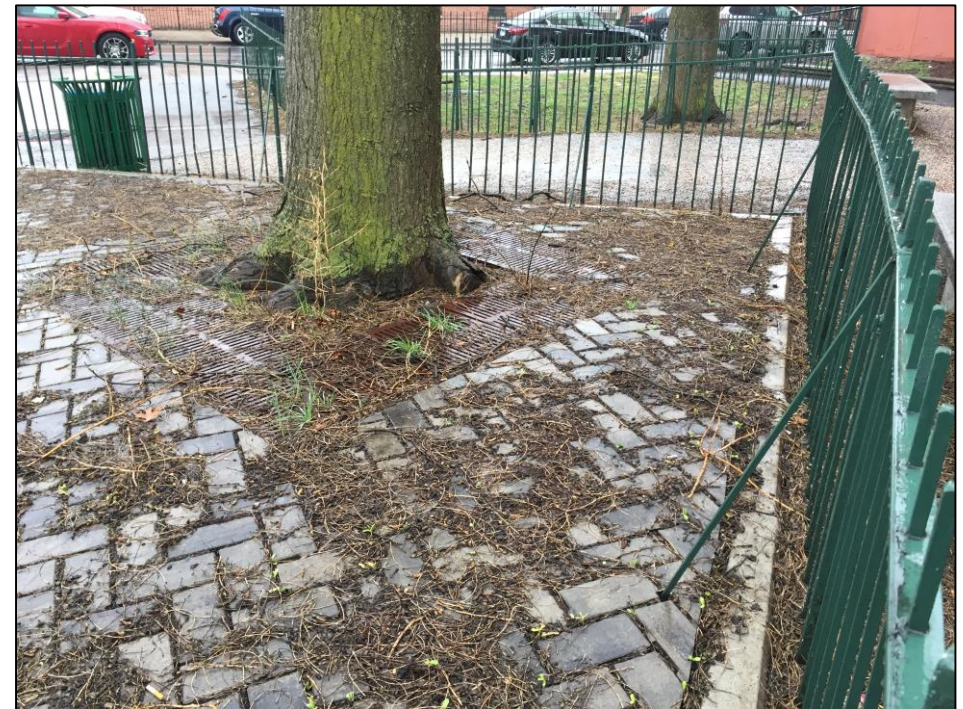
Photo 4: Looking northwest at porous paving installed at Site; twigs, leaves, and twigs present.
