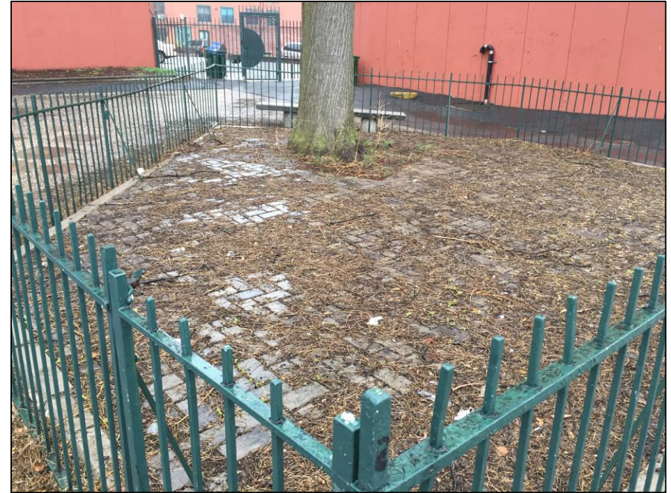
Photo 2: Looking northeast at porous paving installed at Site; twigs, leaves, and twigs present.
