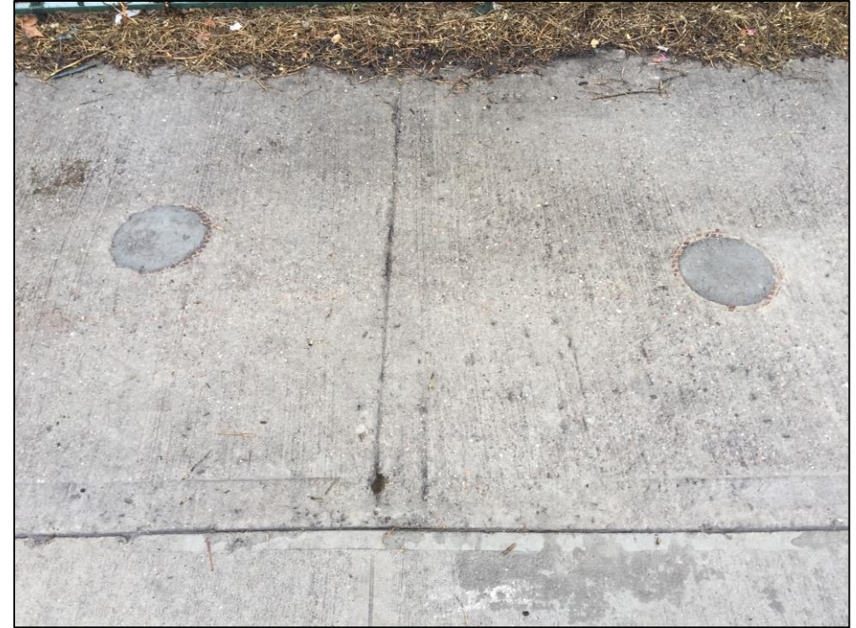
Photo 10: Repaired soil borings/soil vapor sampling locations. No cracks in surrounding concrete sidewalk; no repairs necessary.
