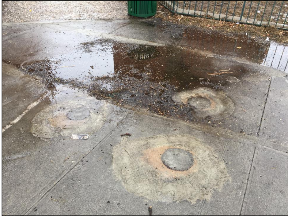
Photo 9: Repaired soil borings/soil vapor sampling locations. No cracks in surrounding concrete sidewalk; no repairs necessary.
